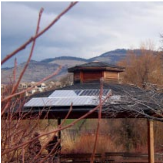
New solar panels on the North Mountain Park pavilion
