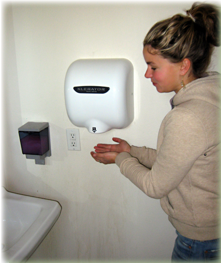
Energy-efficient hand dryers at North Mountain Park
