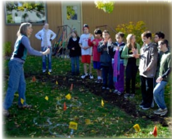
North Mountain Park Stewardship Coordinator, Linda Chesney, leads students in the construction of a rain garden at the Ashland Middle School.
