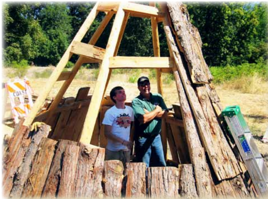
Eagle Scout Kaleb Wagner consults with the Parks Central Division Manager, Jeff McFarland, on the construction of the umma
