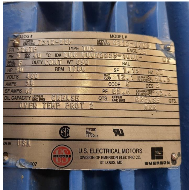
Regional BPS 50 hp pump motor tag
