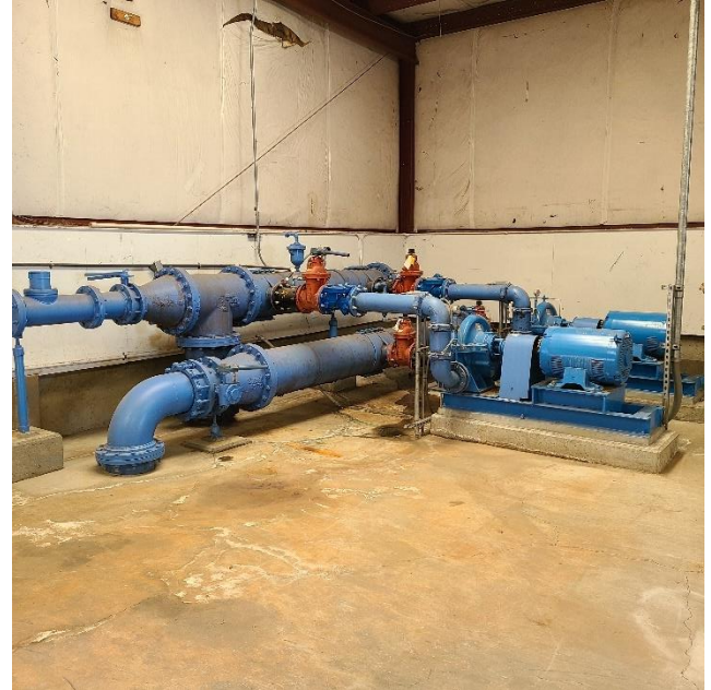
Existing pumps inside the Talent BPS
