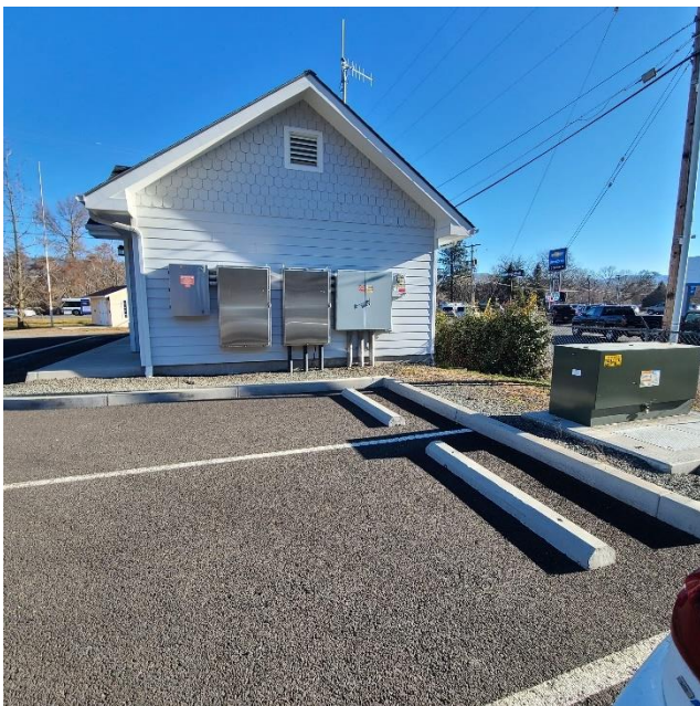
Ashland BPS proposed new generator location
