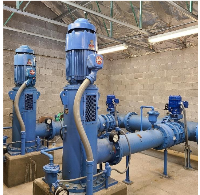
1 of 2 (50 hp) pumps proposed for replacement
