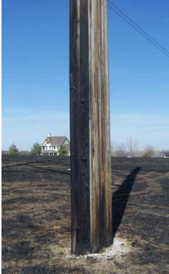
E-LAM® laminated wood structure after a grass fire shows minimal char and less than 1% reduction in strength.
