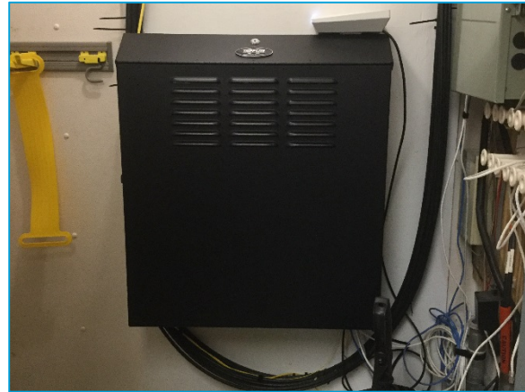
Photo 3-25 – PLC Telemetry Unit
