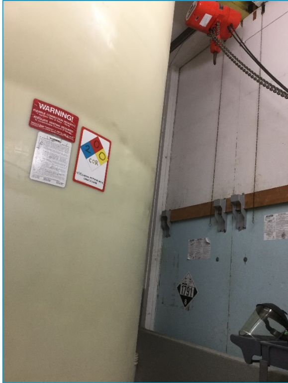
Photo 3-14 – Sodium Hypochlorite Tank and Hoist
