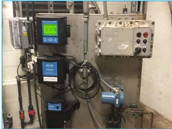
Photo 3-24 – Dual Media Filter #1 Turbidity Meter
