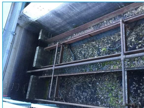
Photo 3-19 – Abandoned Dual Media Filter #7
