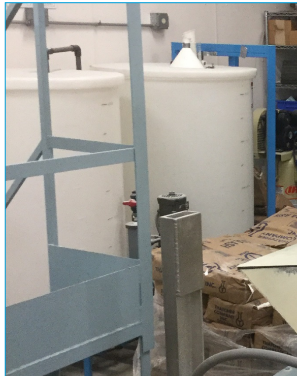
Photo 3-12 – Filter Polymer Aid Feed Tanks
