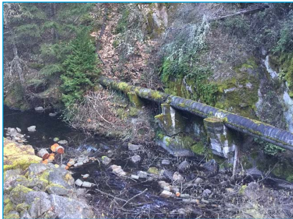
Photo 3-5 – Talent Irrigation District Influent Pipeline
