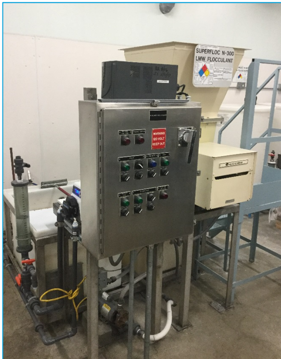
Photo 3-11 – Filter Polymer Aid Hopper and Mixing Tank
