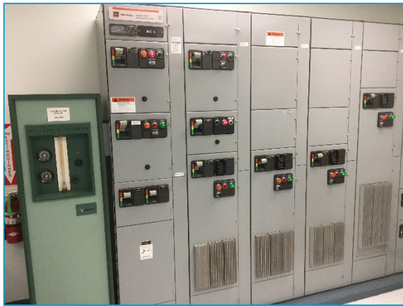
Photo 3-22 – Motor Control Center
