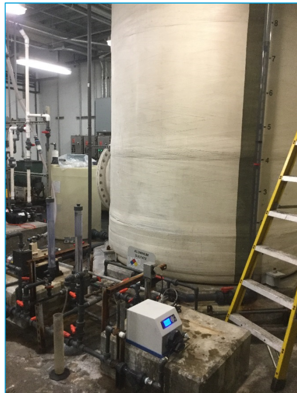
Photo 3-7 – Base and Pedestal of Alum Tank
