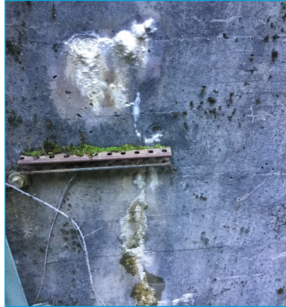
Photo 3-21 – Efflorescence on Exterior Dual Media Filter Wall
