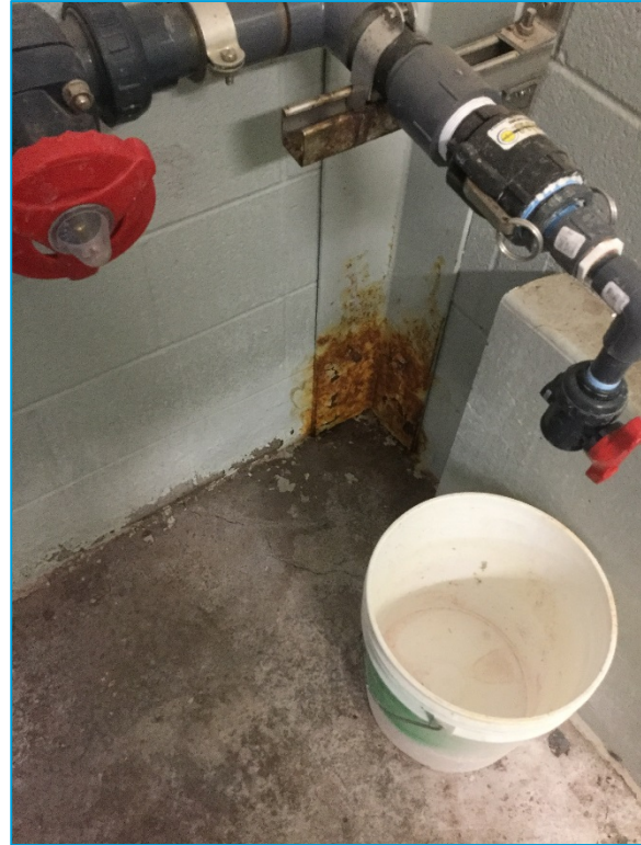
Photo 3-15 – Corrosion in Chlorine Building
