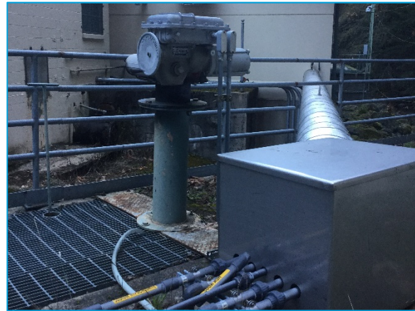
Photo 3-4 – Influent 36-inch Butterfly Valve
