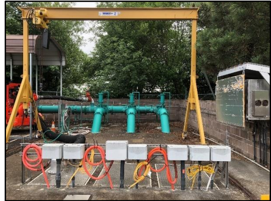
Ashland Creek Lift Station (June 16, 2020)
