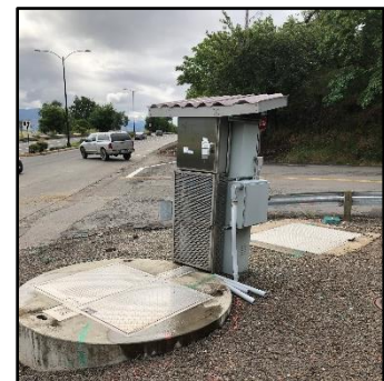
North Main Lift Station (June 16, 2020)
