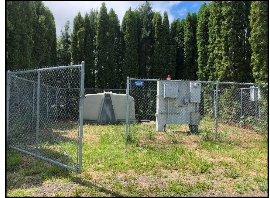
Kestrel (North Mountain) Lift Station (June 16, 2020)
