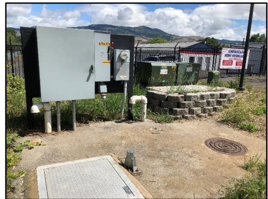
Shamrock Lift Station (June 16, 2020)
