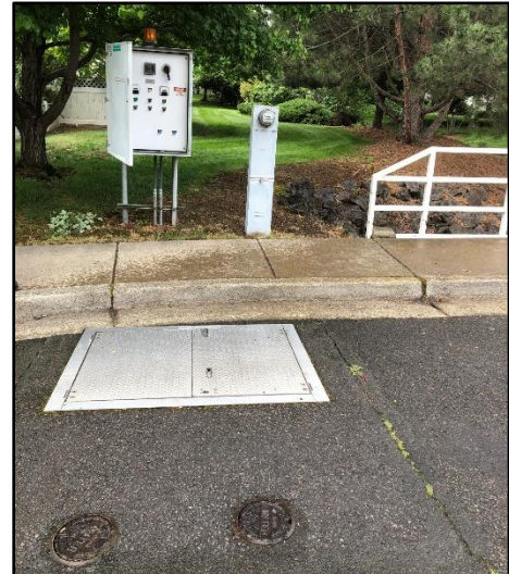
Creek Drive Lift Station (June 16, 2020)
