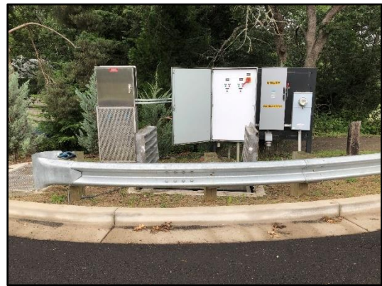
Grandview Lift Station (June 16, 2020)
